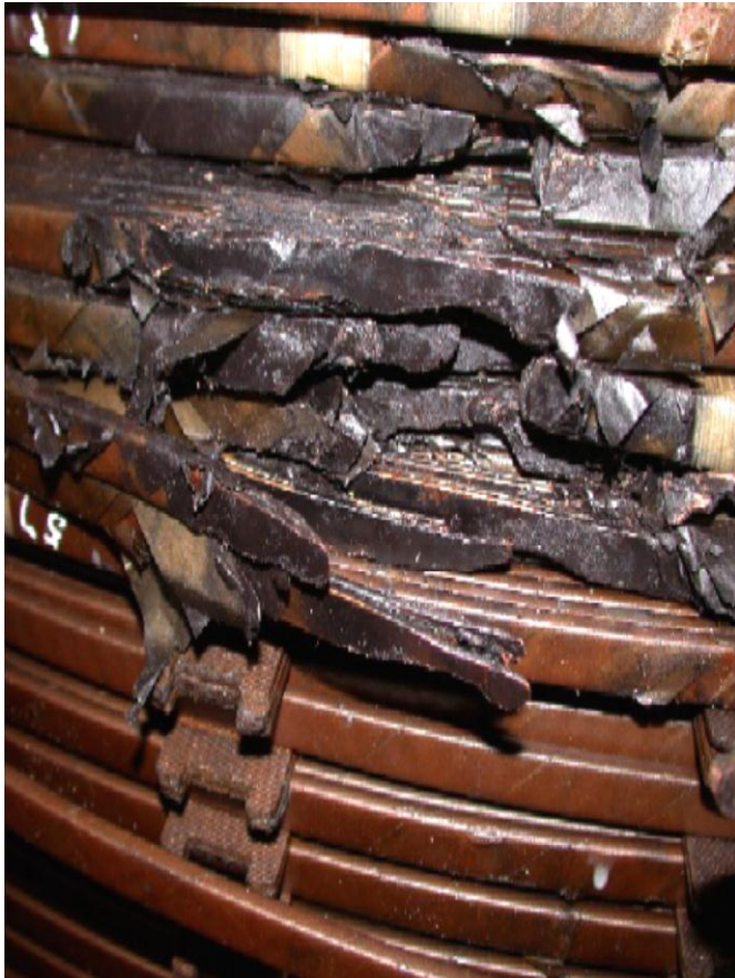
Station 3 Gen Transformer 4 HV winding failure
