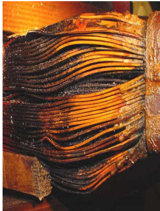
Station 3 Gen. Transformer 5 evidence of overheating
