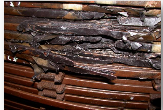
Transformer damage from moderate solar flare – S. Africa
